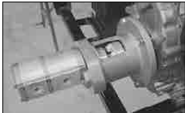
Fig 17 - Hydraulic pump over shaft
