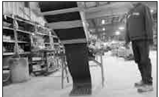
Fig 166 - Belt under hopper
