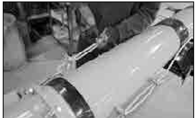
Fig 181 - Cables attached to hopper end
