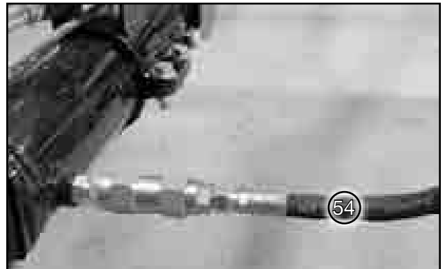
Fig 92 - Fittings to the hydraulic cylinder
