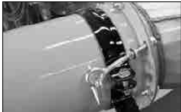
Fig 178 - Eye bolts in discharge flange
