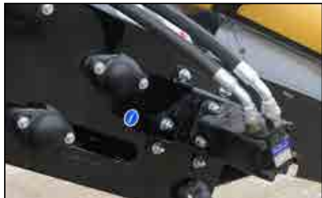
Fig 61 - Conveyor belt hydraulic drive motor
